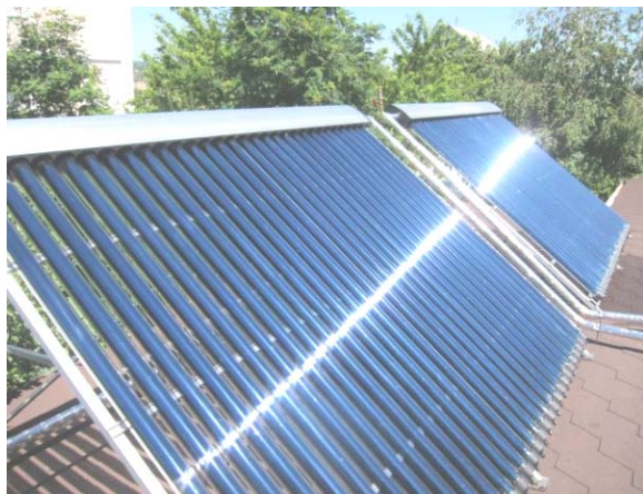
Fig. 11. Solar collector on the building roof
